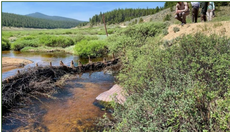
Photo by Jackie Corday, a “starter dam” installed to protect a road culvert.
