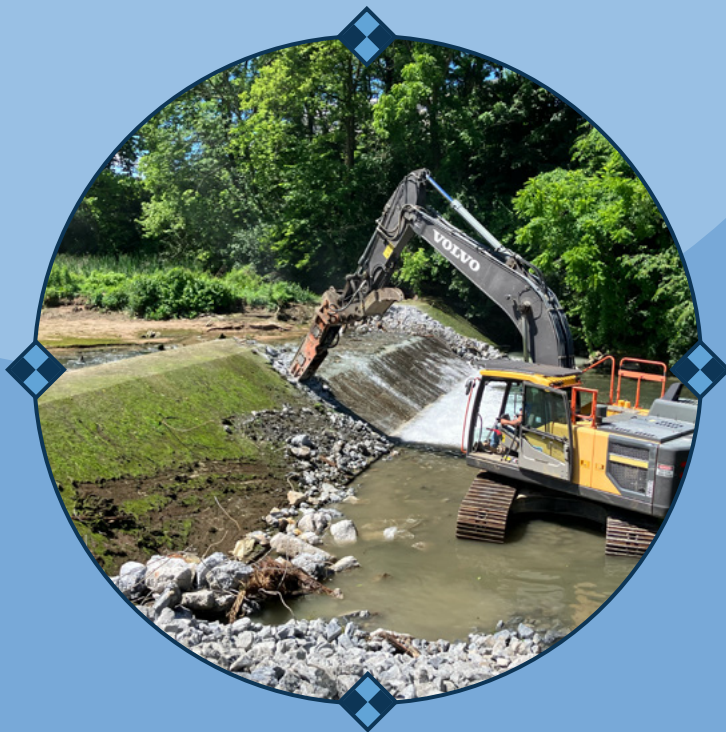
Deconstruction of the Van Reed Paper Mill Dam in Reading, PA, was completed in 2022. The project reconnected the river corridor for fish and wildlife and restored native vegetation along the riverbank, among many other benefits. Credit: Kleinschmidt Associates
