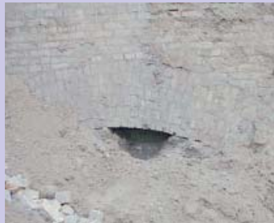
Early excavation of an original brick arch over Minneapolis Mill tailrace tunnel.
