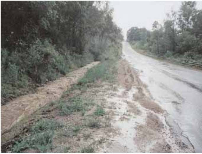
Roadside erosion due to flooding (Photo: Patricia Pennell)
