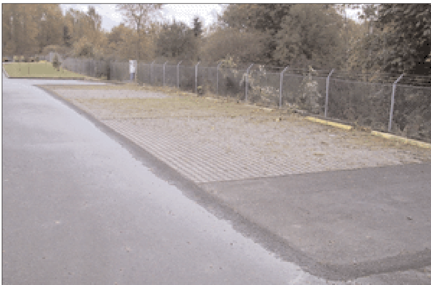
Block Paver and Permeable pavement being tested at the University of Washington (Photo: Center for Water and Watershed Studies)
